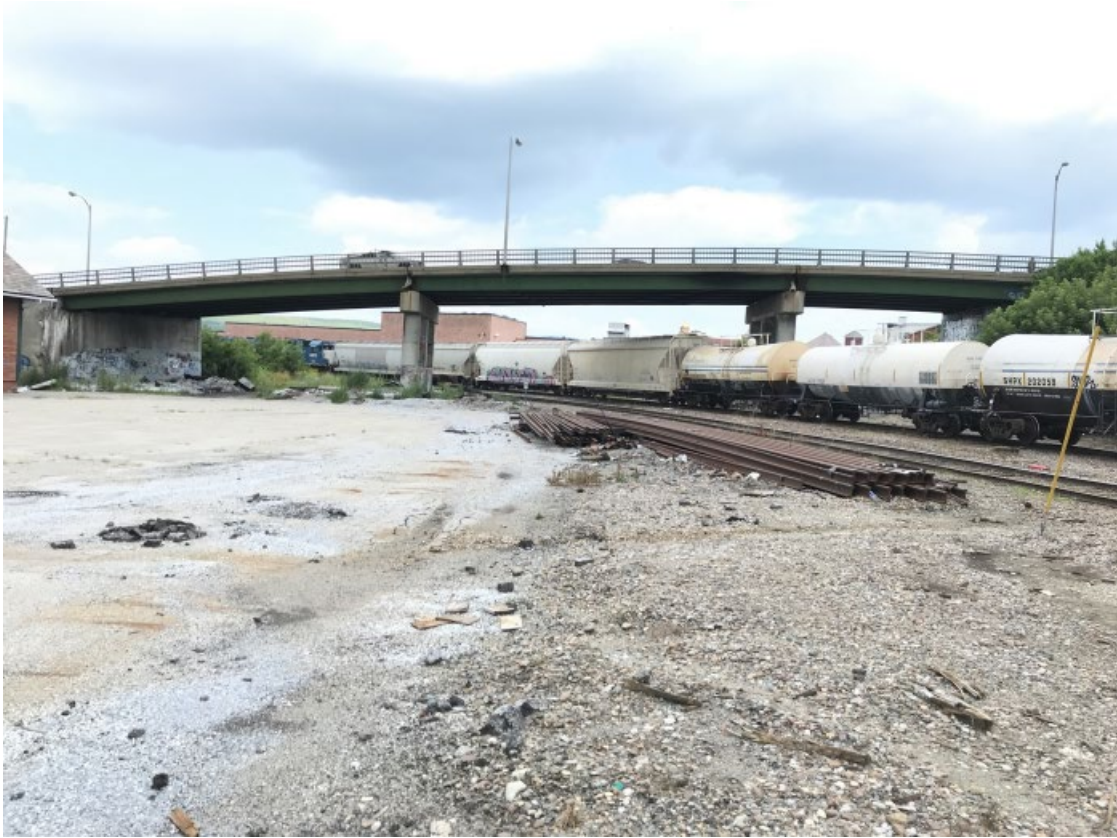
Figure A1: Overall View. Rutland City, Bridge #27, River Street. Photo from 07/21/2022 inspection.
