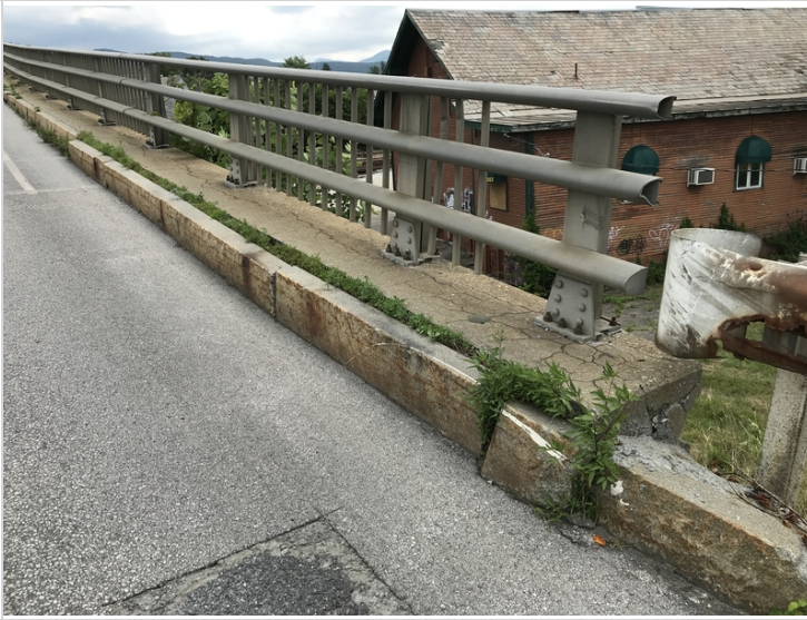
South rail damage, missing ballasters & displaced curbing at West approach
