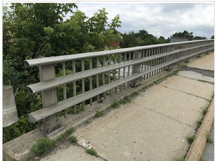
North rail damage West approach
