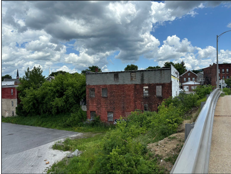
Figure 3. Overview facing northeast towards Strongs Ave with paved loading bay and commercial property.
